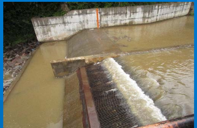
Prototype of the first advanced drop intake in Nepal (5.1MW Mai Chhedi)
